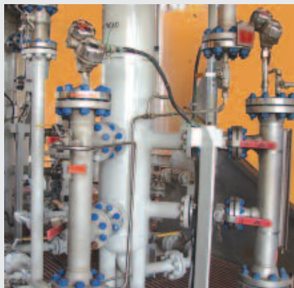
Oil & Gas Platform
