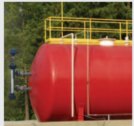
Fuel Oil Storage
